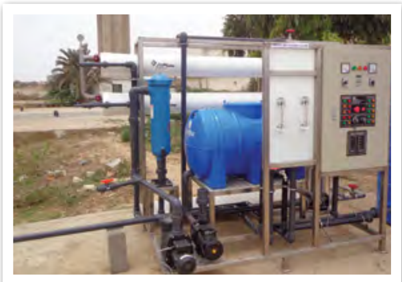
We're powering our filtering plants by renewables (Photo: © Pak Oasis)
